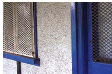
Figure 33 Chrysotile pebble-dash exterior wall coating
