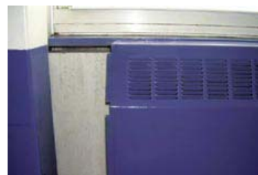
Figure 19 AIB behind school radiator unit
