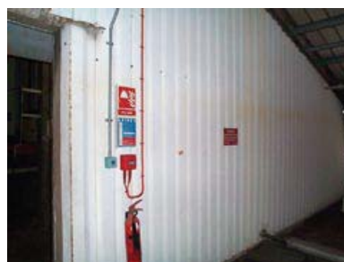
Figure 38 Chrysotile/bitumen coating under metal cladding
