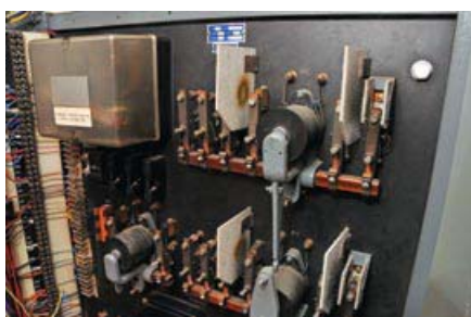
Figure 50 Open electrical switchboard with asbestos flash guards
