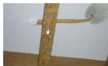
Figure 25 Chrysotile paper on strawboard ceiling panels
