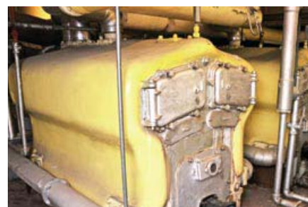
Figure 13 Amosite lagged boiler with hard plastic coating
