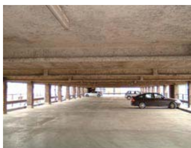
Figure 7 Sprayed limpet on car park roof
