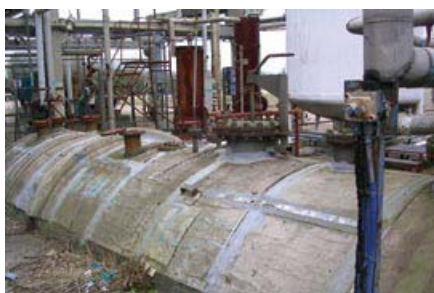
Figure 12 Lagging on large petrochemical vessel
