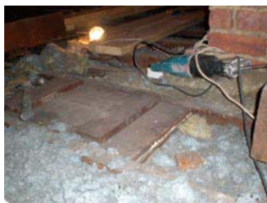
Figure 6 Loose asbestos used as loft insulation
