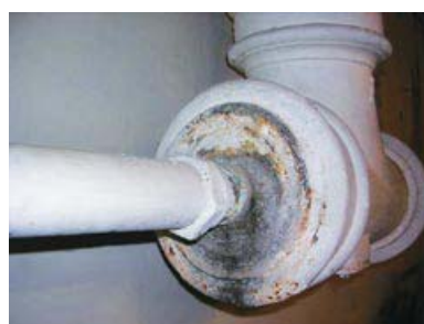
Figure 30 Amosite and chrysotile packing on waste pipes
