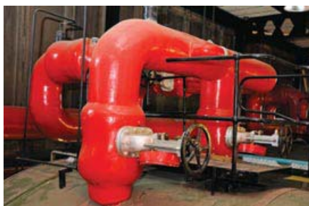
Figure 48 Asbestos-insulated supply pipes
