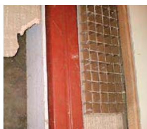
Figure 21 AIB column fire protection in CLASP building
