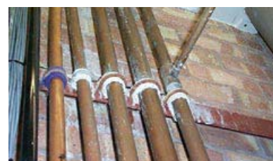
Figure 29 Chrysotile cloth on pipes
