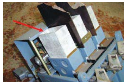
Figure 49 Electrical switchgear with asbestos flash protection
