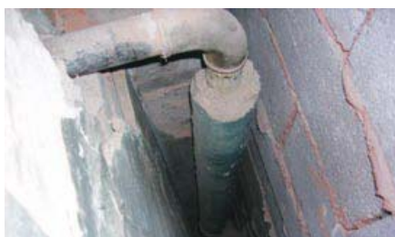
Figure 9 Lagged pipe in wall cavity
