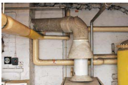
Figure 34 Asbestos cement boiler flue
