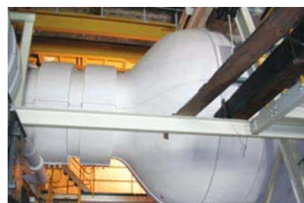
Figure 51 Vessel clad in amosite insulation
