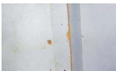
Figure 24 Chrysotile paper on fibreboard boxing
