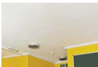
Figure 36 Asbestos textured coating on ceiling
