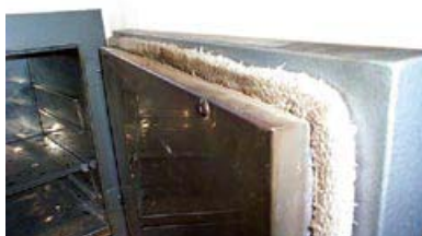
Figure 26 Asbestos rope seal on drying oven
