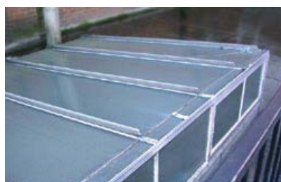
Figure 31 Chrysotile string on skylights
