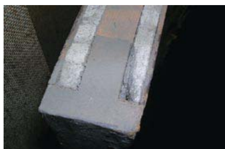
Figure 14 Asbestos panels inside fire door
