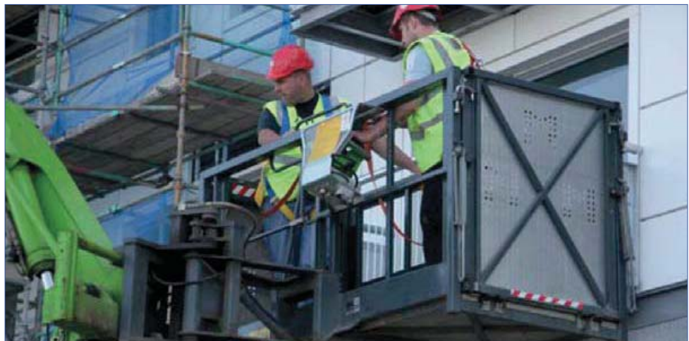
Figure 19 Integrated working platform
