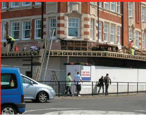
Pedestrians are at risk from falling tools and materials, and workers are at risk of falling
