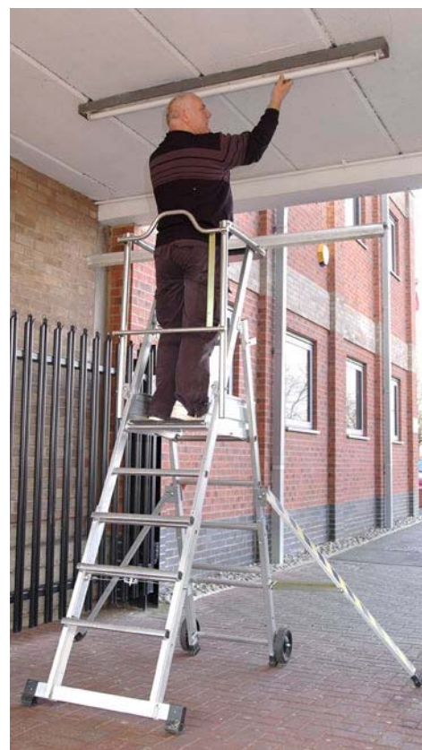
Figure 22 Working platform stepladder
