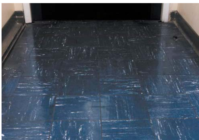
Figure 48e Asbestos-containing vinyl floor tiles
