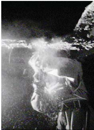
Figure 7.1 Uncontrolled dry stripping
