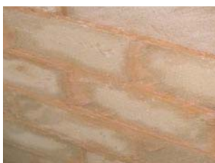
Figure 7.26 Remnants of asbestos on breeze blocks
