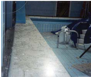
Figure 1.7 Uncontrolled removal of asbestos
