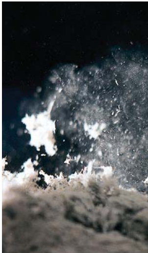
Figure 1.1 Asbestos fibres being released from lagging
