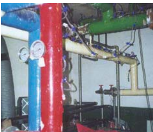
Figure 7.9 Good practice: Wet injection on pipework
