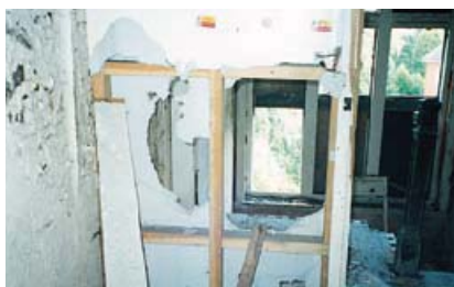
Figure 7 Asbestos insulating board wall panels badly damaged
