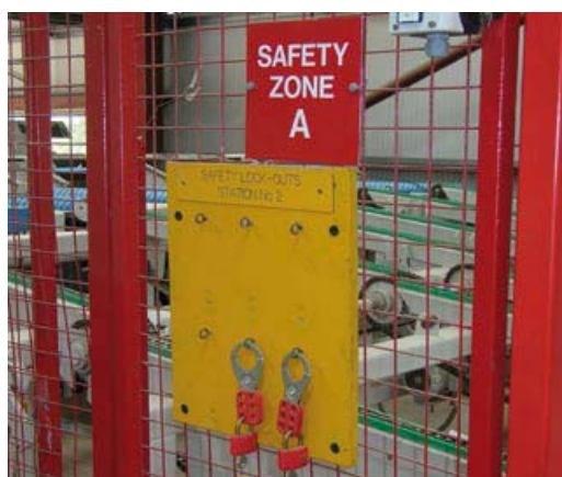
Figure 30 Safety lockout station
