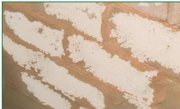
Figure 6.5 Remnants of asbestos on breeze blocks
