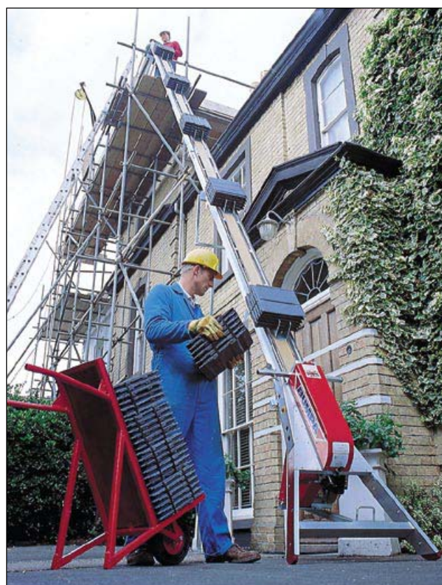
Figure 5(b) Domestic hoist
