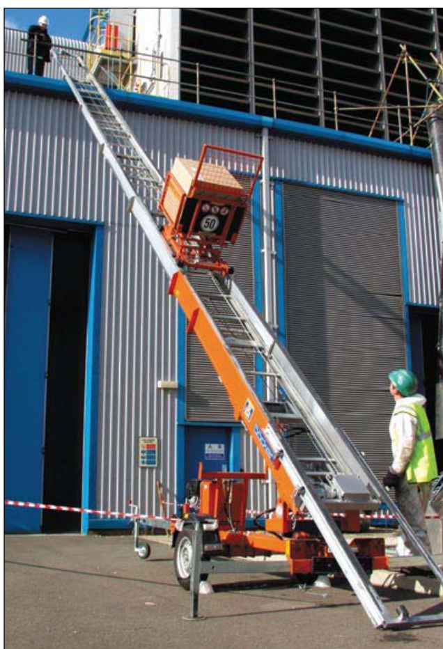
Figure 5(a) Industrial hoist (Images courtesy of HSS)
