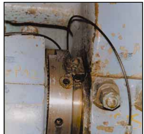
Poor standards of repair during maintenance
